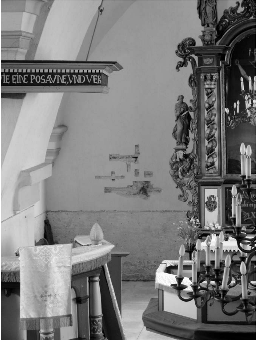
Fig. 4. Discovering the aumbry niche in the eastern wall of the chancel - plaster partly removed from the masonry (in the middle of the photo). Photo by Villu Kadakas.
