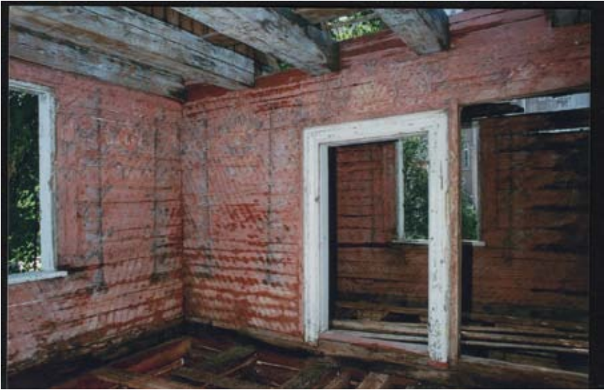
Fig. 1. Liepāja, 11/13 Baznīcas Street. Second floor painted colonnade on wooden beams. 1740s–1750s. Photo by Juris Zviedrāns, archives of the Architectural Investigation Group Ltd.
