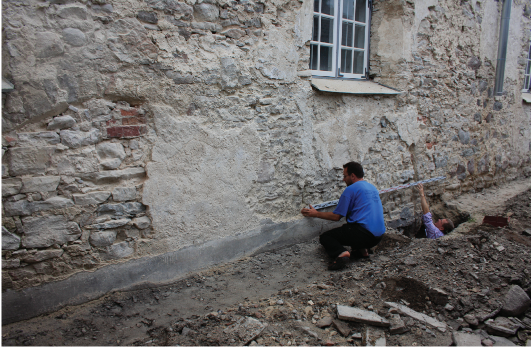
Fig. 10. St John's Church in Haapsalu. Measuring the former entrance to medieval granary. Jn 10. Jaani kirik Haapsalus. Keskaegse aidaava sissepääsu mõõdistamine. Photo / Foto: Erki Russow
