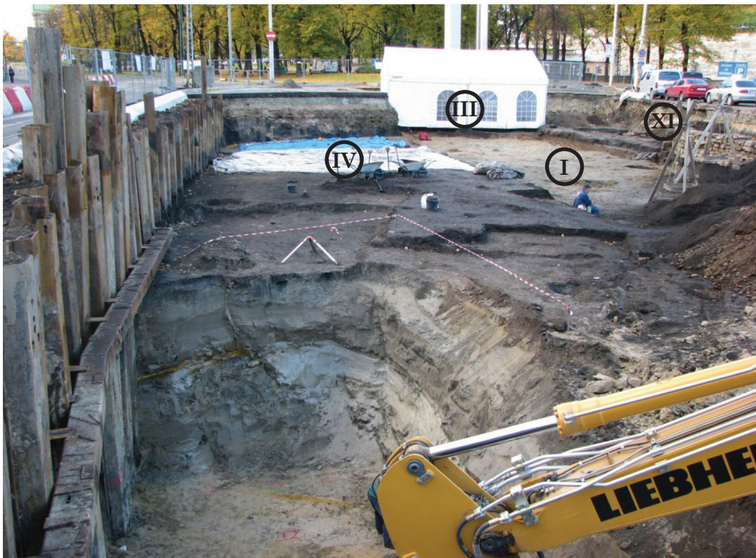
Fig. 2. Excavation plots IV, I, III and XI at Vabaduse Square. View from the south-west.
