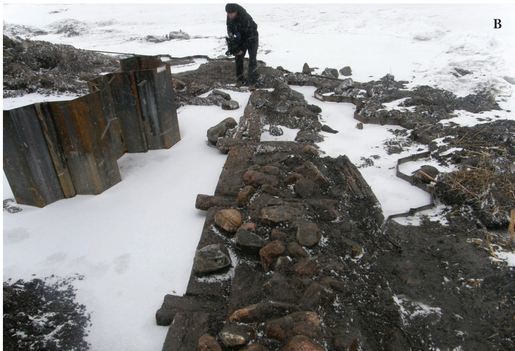
Fig. 6. A – construction of the second half of the 18th c bank fortifications, B – the 18th c bank construction at the corner of the southern bank of the moat and the western bank of the tributary moat.
