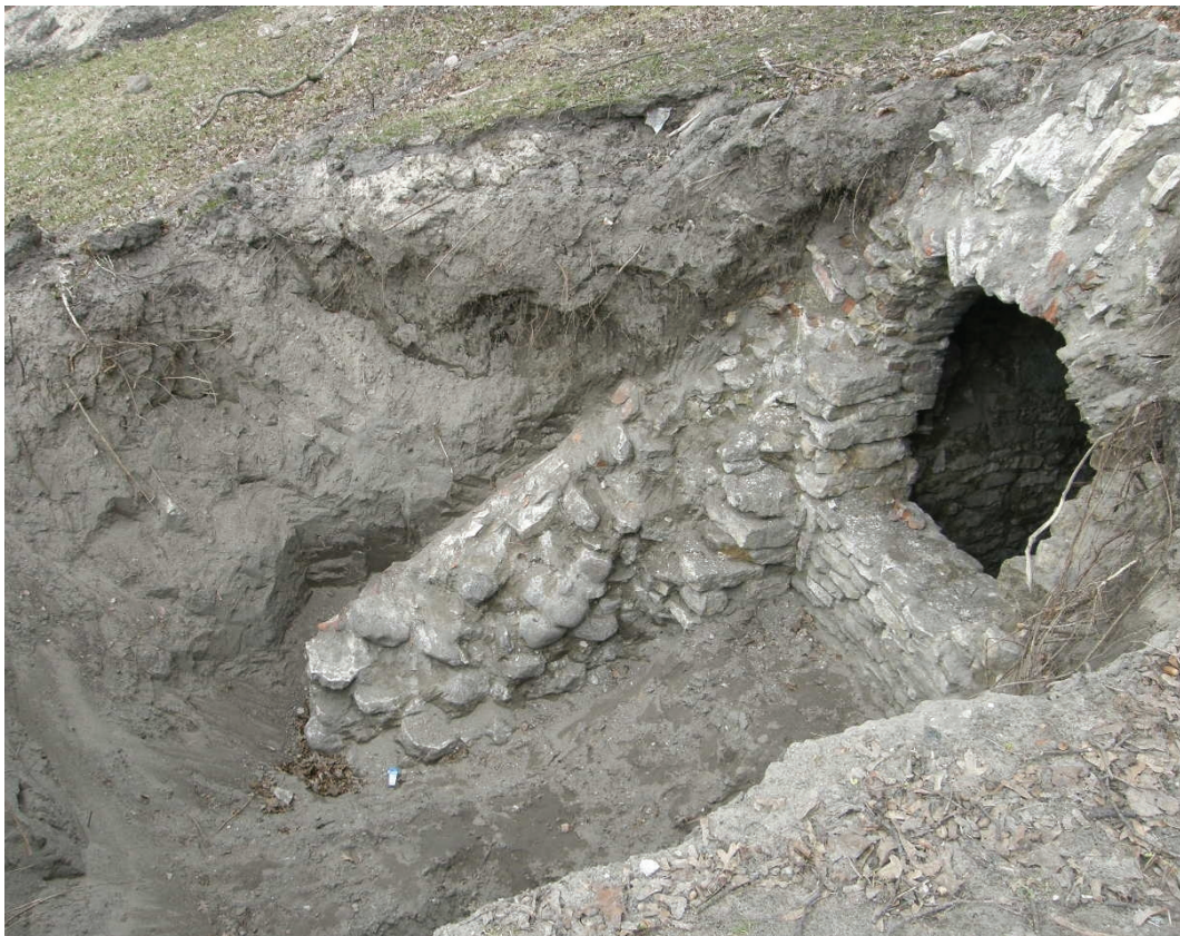
Fig. 8. Supportive walls in front of the outer side orifice of the sally port.
