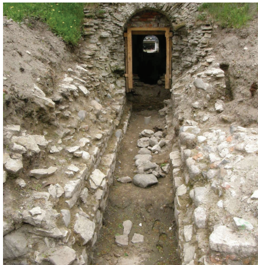
Fig. 9. Supportive walls in front of the sally port by the inner side of the earthen rampart.
