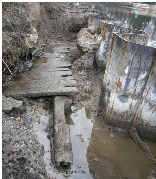
Fig. 10. Supportive construction, composed of horizontal planks and baulks at the southern face of the bastion Luna.
