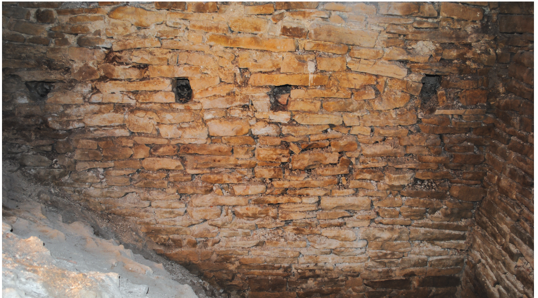
Fig. 4. Holes discovered in the northern wall of the church.
