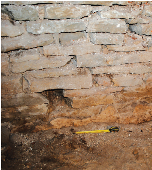
Fig. 1. Holes for beams in the southern wall of the church and remnants of plaster revealed under the holes.
