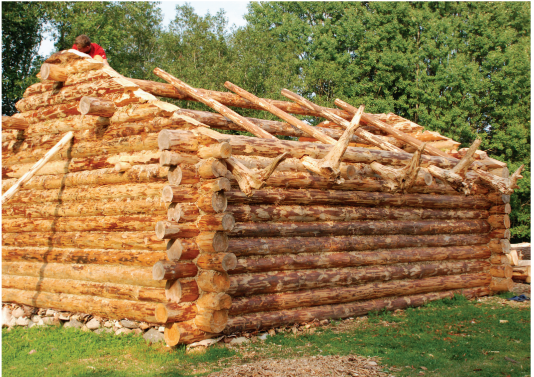
Fig. 5. The rafters are placed on the last but one (the ninth) log.
