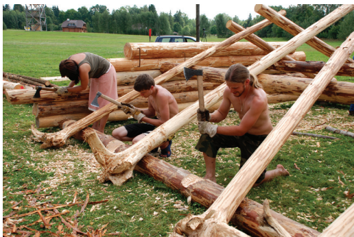
Fig. 6. The support construction of the roof was prepared separately from the house.
