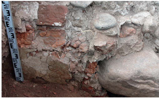
Fig. 6. Test pit 2. Remains of the southern fragment of plaster on the outer face of the eastern wall of the chapel and springing of the vaulted arch.
