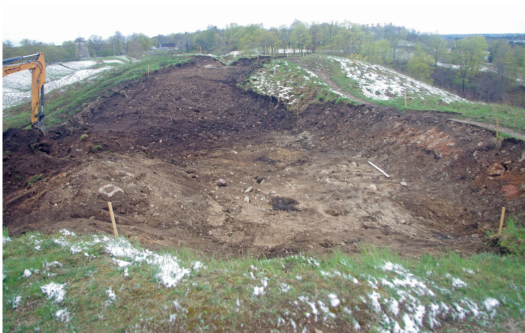
Fig. 3. Stripping the topsoil on the SW bastion. Photo from the north. The rectangular depression on the foreground and higher bastion in the rear. The dark and burnt soil layer covers the slope of the bastion. A burnt clayish layer, mixed with burnt logs and stones from the western wall at the right side of the photo.
