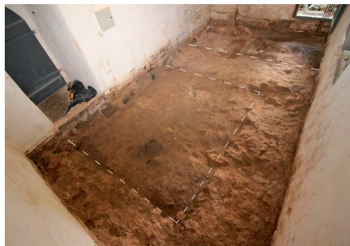
Fig. 4. Interior of the sacristy after excavations in 2017: contours of the foundations of the medieval sacristy are marked in a dashed line. View from the north-eastern corner.
