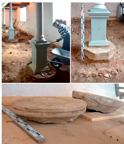
Fig. 4. Details of the medieval pillars in Rannu church from the southern aisle. a – unearthened pillar details in situ, b – the easternmost pillar fragment in situ, c – the pillar bases after removal.
