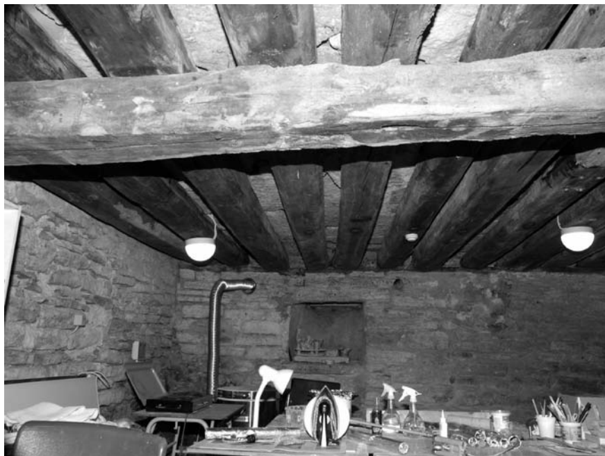
Fig. 13. Extra beam supporting the beams in the southern basement. Photo by Heidi Tooming.
